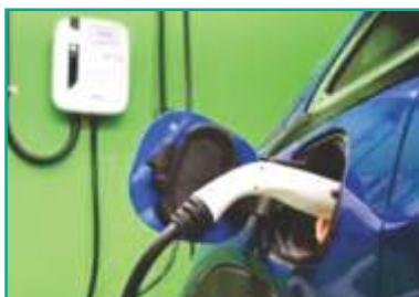
Electric Vehicle Charging (120 kW DC)
