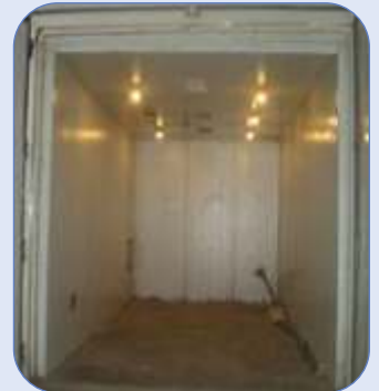
Walk- in Hot & Cold Chamber
